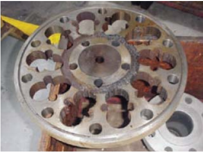
H. Flow divider was gunked up, corroded and inoperable
